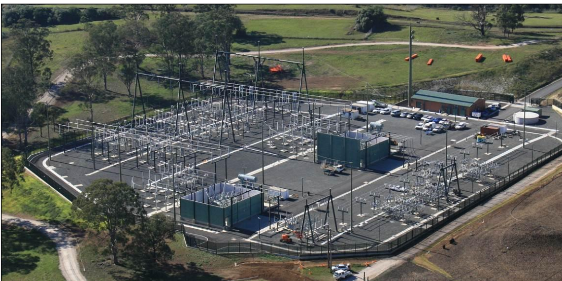
Figure 3-10 TransGrid's 330 kV Macarthur Substation in western Sydney
