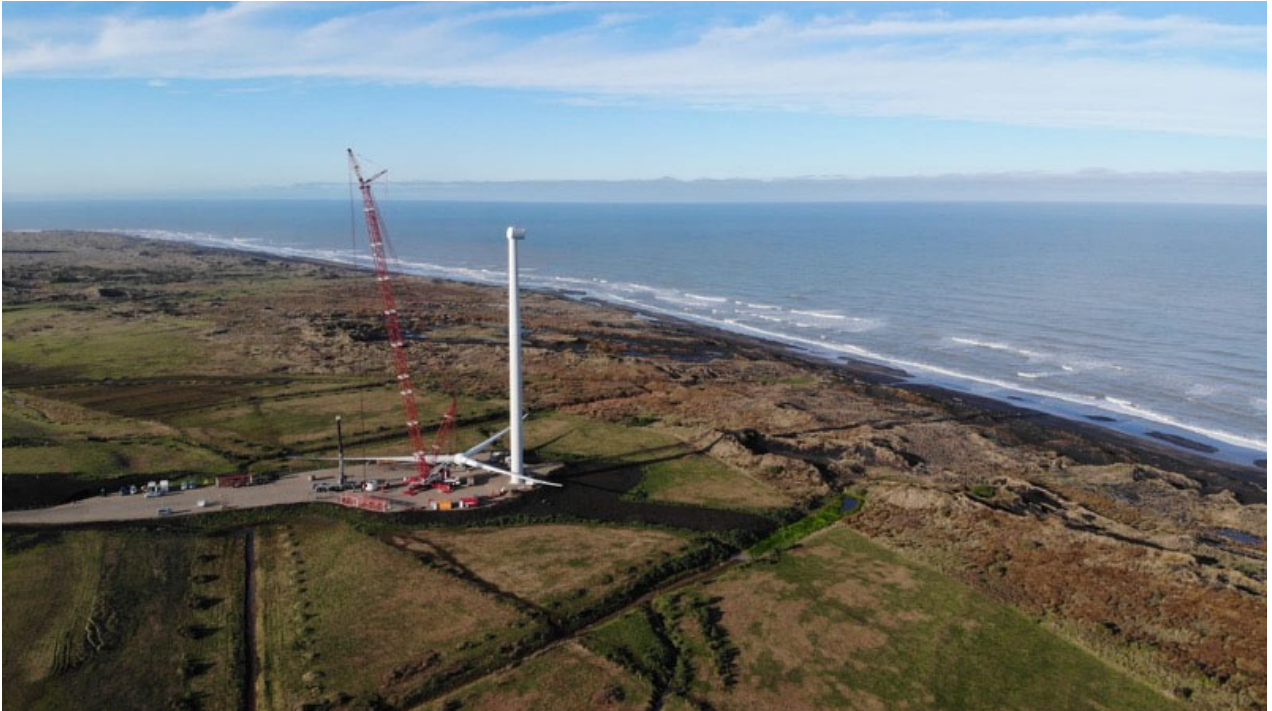
The rotor assembled and waiting for the wind conditions to allow lifting.
