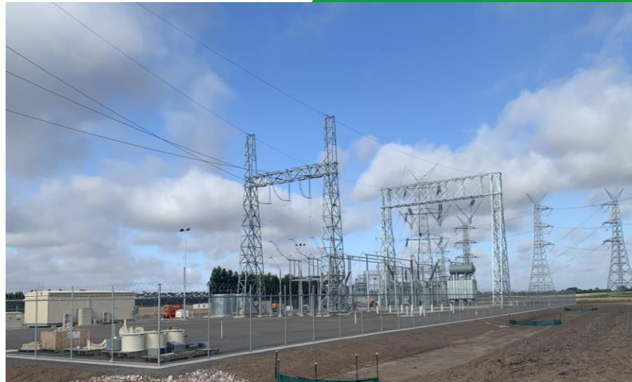
The completed substation
