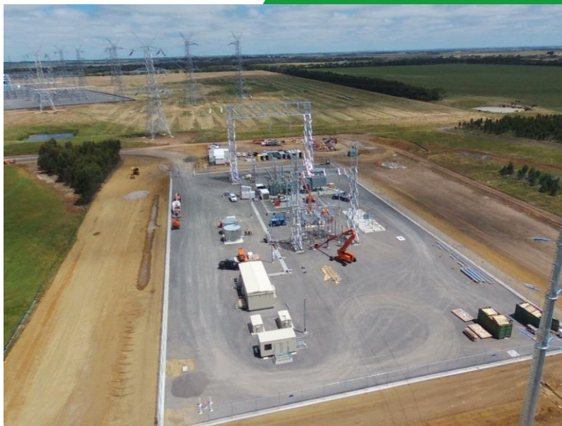
The completed substation
