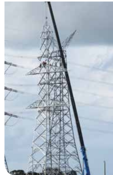
Lattice transmission line tower (approximately 68 metres tall).
