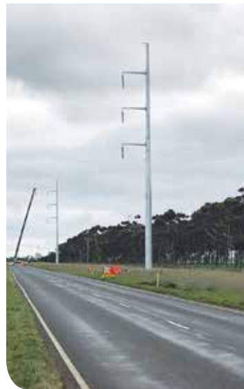
Transmission line poles (approximately 40 metres tall) in Mortlake-Ararat Road.
