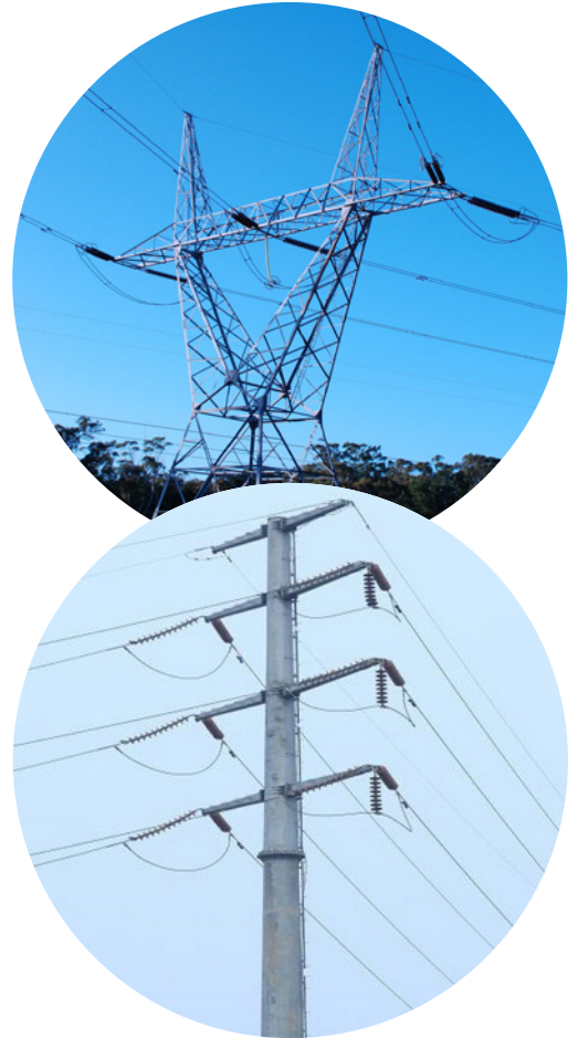
Top: Flat top strain tower Bottom: Double circuit strain pole
