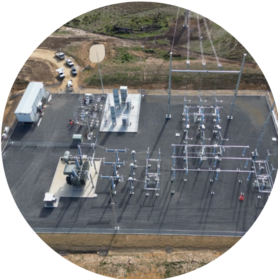
Figure 9: The southern substation
