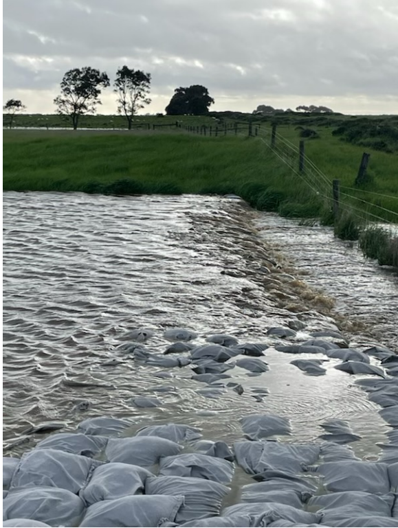
Photo 3. Installed sandbag block after 70ml of rain in October 2022
