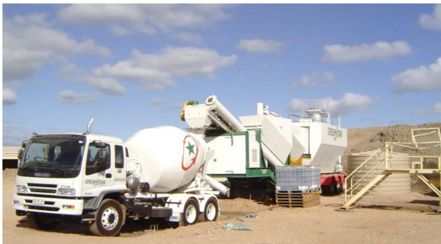
Photograph 2-4 Typical Temporary Concrete Batching Plant
