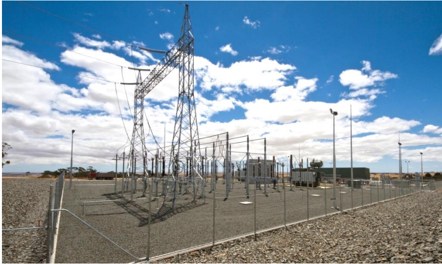
Photograph 2-1 Typical 220/33kV Substation
